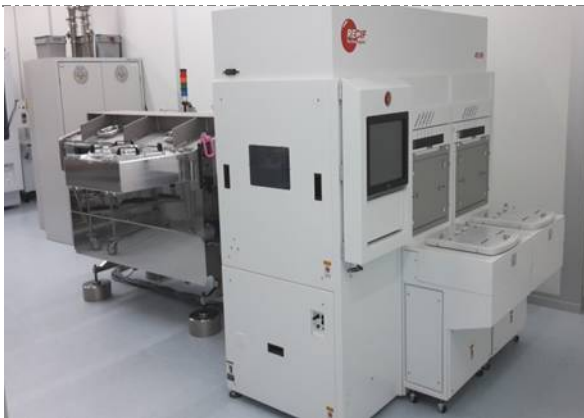
RECIF 450mm EFEM installed in imec clean room
